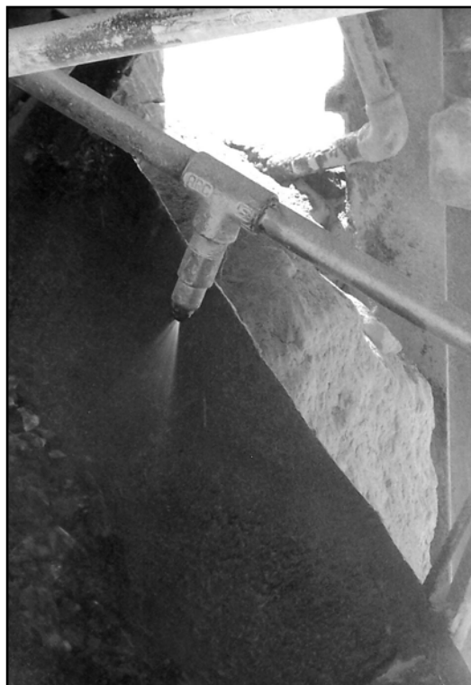
Picture 10: water spray nozzle above chute. Source: Occupational Knowledge International
