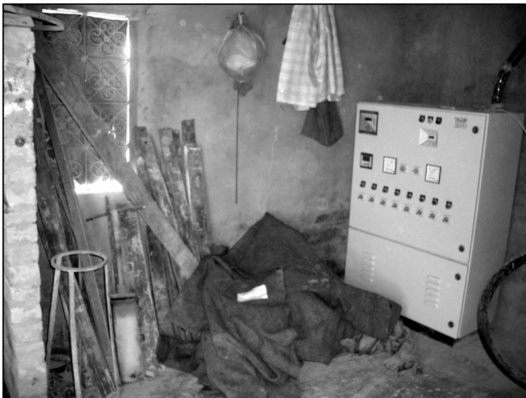
Picture 14: flammable material in the electric room is a fire hazard
