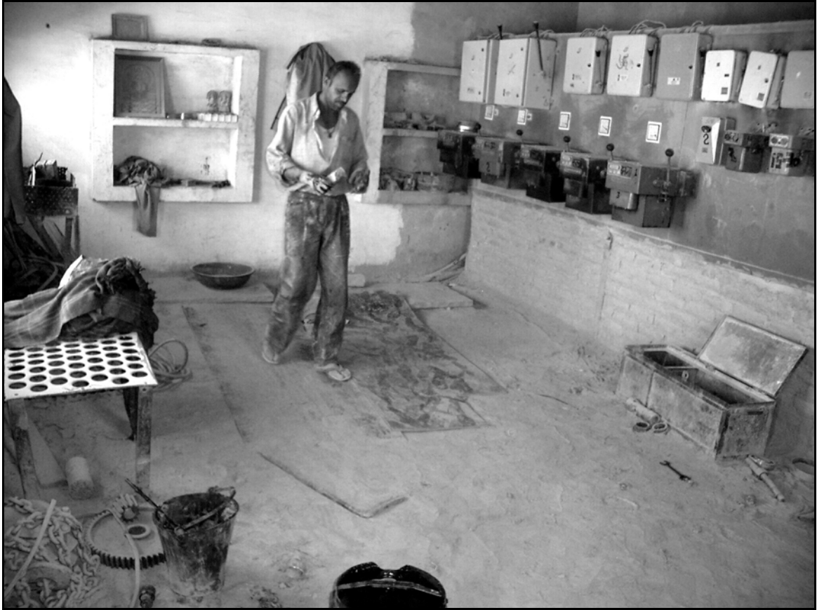
Picture 5: electrical room used for storage and rest
