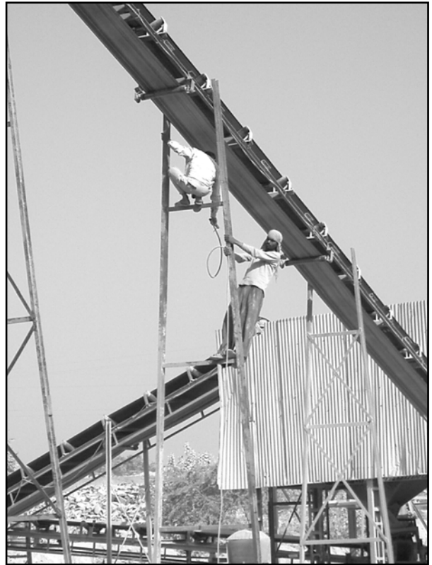
Picture 4: repairing the conveyer belts without safety harness or fall protection
