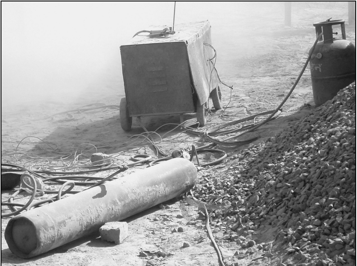
Picture 7: compressed welding gas cylinder (foreground) together with LPG gas tank (right side) close to a power generator on open, hand-twisted electrical cable connections (center)
